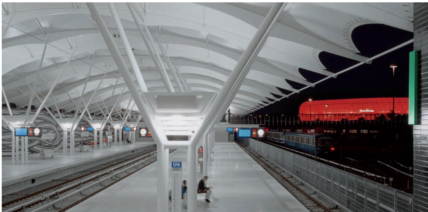
OSRAM has installed 150 Endura lamps in the 14 support pillars for the roof structure over the Fröttmann station at the Munich football stadium. The luminaries are completely hidden from the view of passengers.
